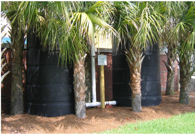
Two 1,550 gallon cisterns are used to harvest rainwater that has filtered through the Perry Construction Yard green roof at the University of Florida in Gainesville
